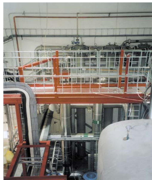
Water/Water heat exchanger for heat extraction and feeding into the district heat system: 5.8 MW • 75 °C
