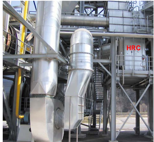
Water/Gas Heat Exchanger for preheating of combustion air: 80,000 m 3 /h • 1.4 MW
