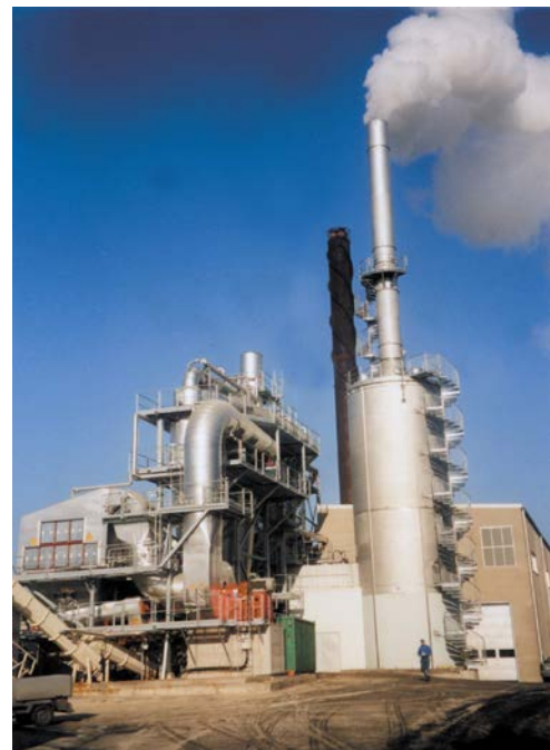
Pellet drier with wet absorber, wet electrostatic precipitator and water/water heat recovery system
